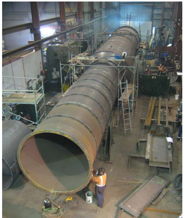
Boiler stack – Dairy Trust Southland
