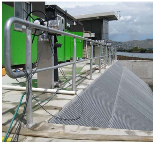
Guardway hand railing – Ocean Outfall Pump Station
