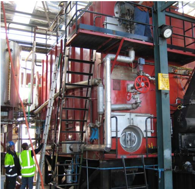
6MW coal boiler – Juice Products Timaru
