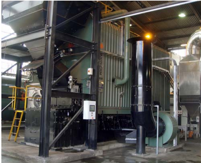
8MW coal boiler – Waiouru Military Camp
