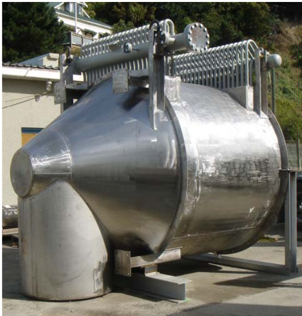
Steam superheater – Dunedin fertiliser plant
