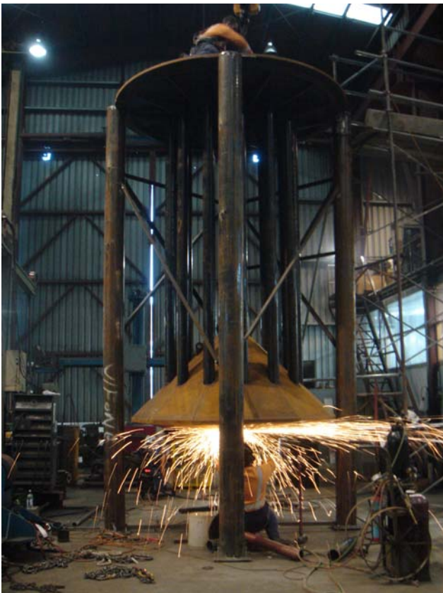
Eductor tube – Bromley Wastewater Plant
